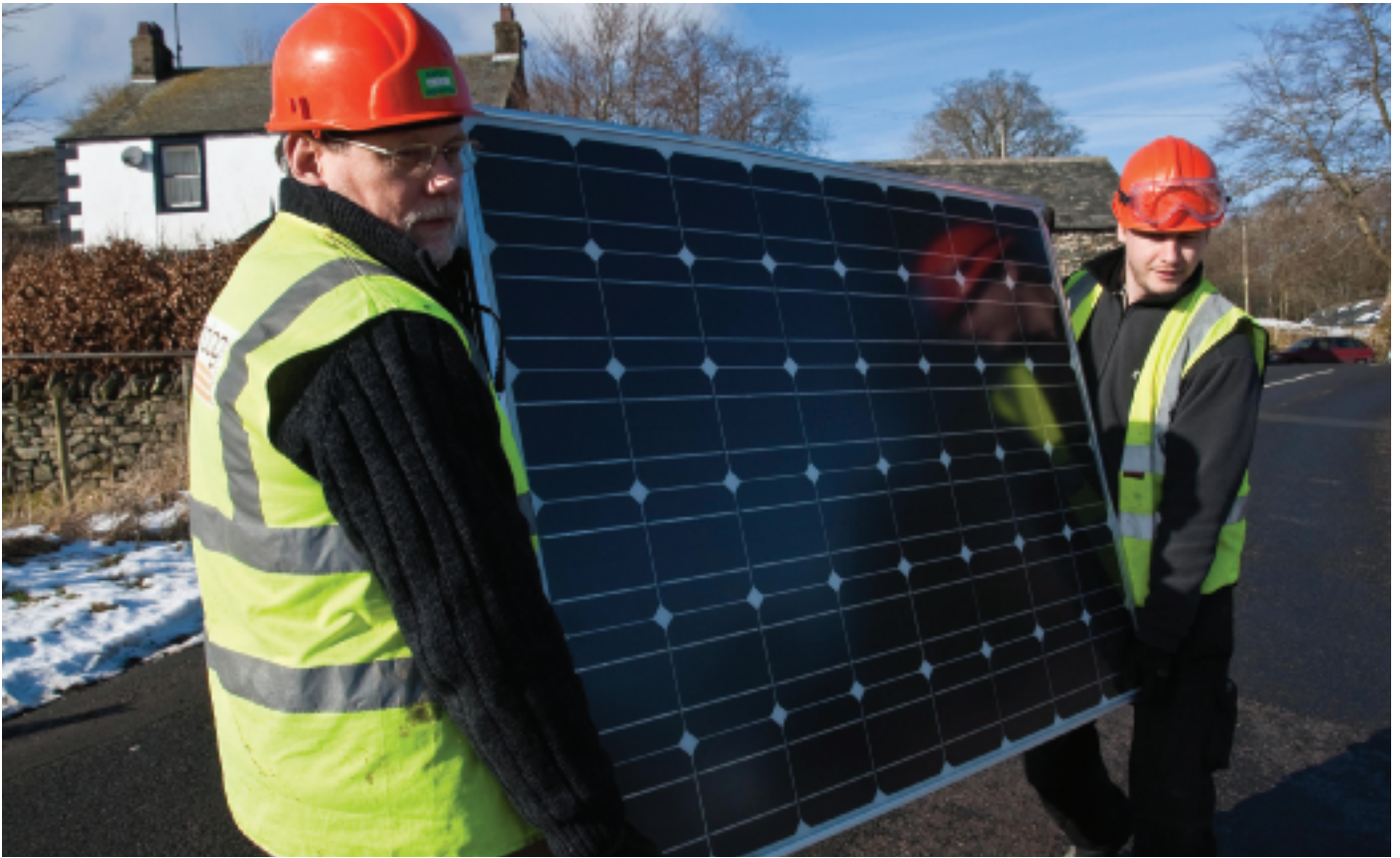
Installing solar panels thanks to Foundation, a Climate Fund for the Northwest
