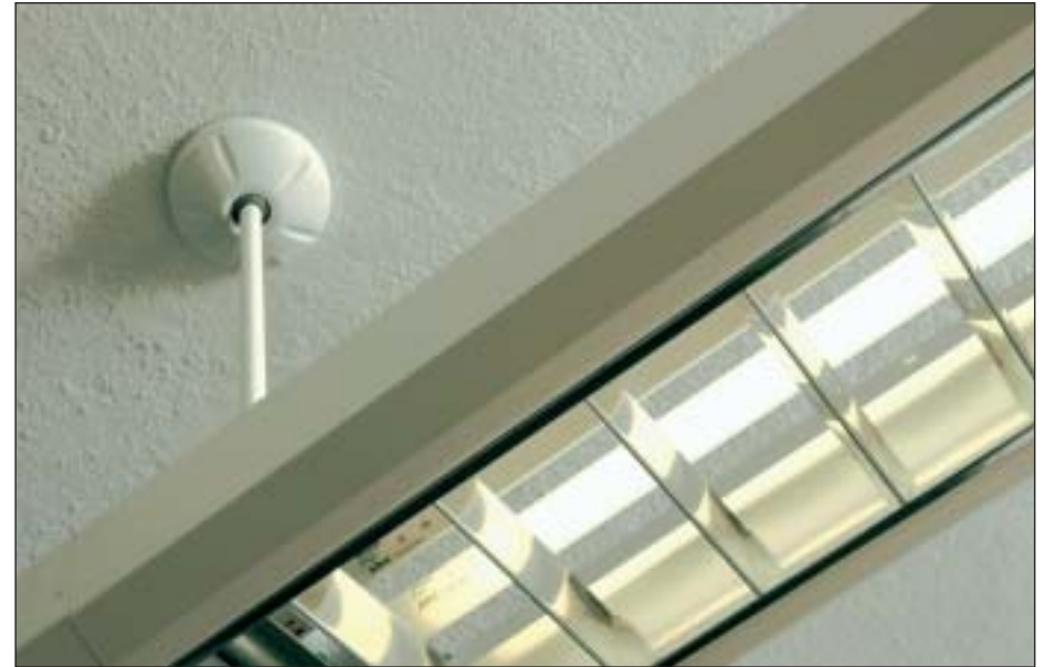
The UNH Energy Office has installed more than 30 energy efficiency projects that include lighting retrofits, heating controls, and replacement of outdated equipment. Energy efficient light fixtures (above), large windows, and glass office doors, were installed in the Nesmith Hall renovation, the home of the Office of Sustainability Programs.
